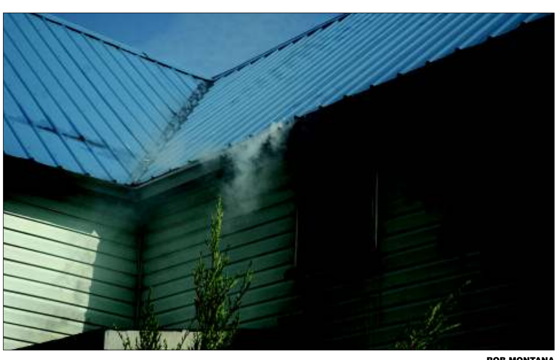
Smoke and water flows from under the roof of the home of Gene Garrison at 5116 Henry Jenkins Road in Hartsville Saturday morning. ROB MONTANA
